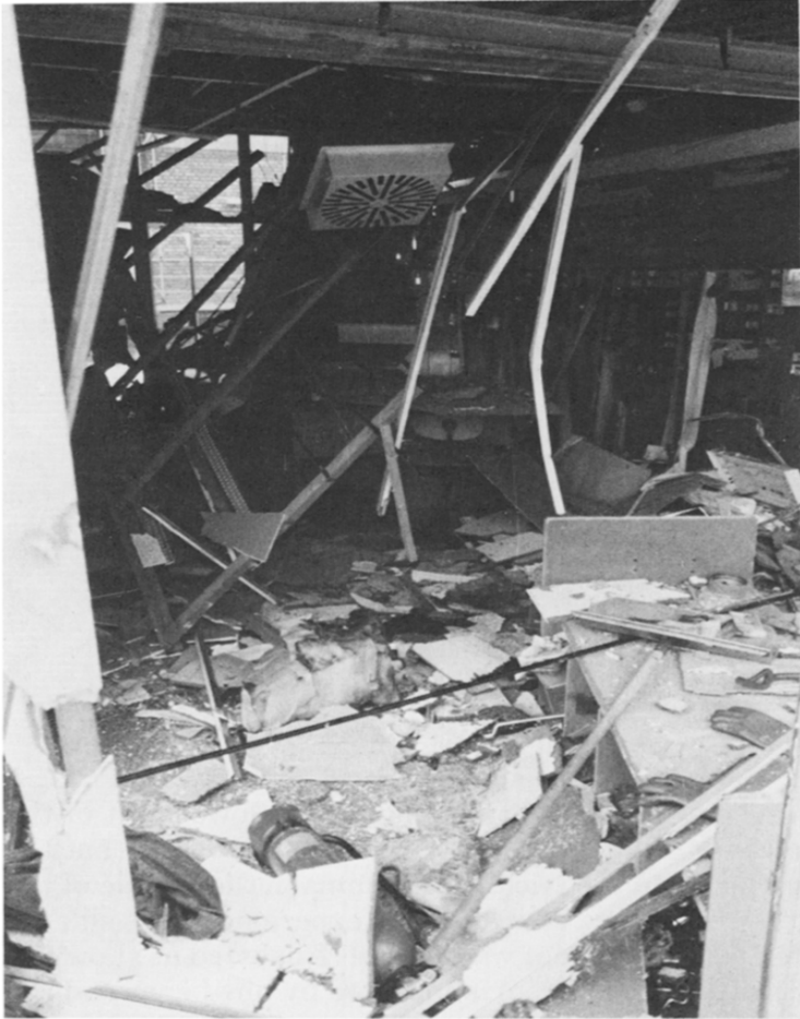
Fig. 11. Destruction in control room of adjacent plant.
